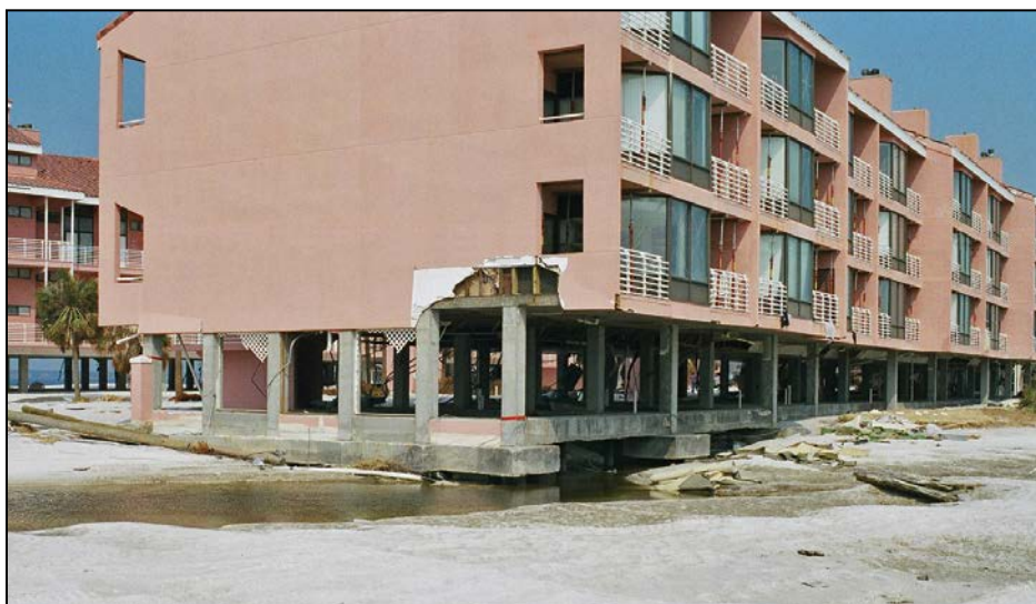
Figure 17: Grade beams that were exposed to flood forces during hurricane-induced scour; grade beams must resist flood, wave, and debris loads when undermined
