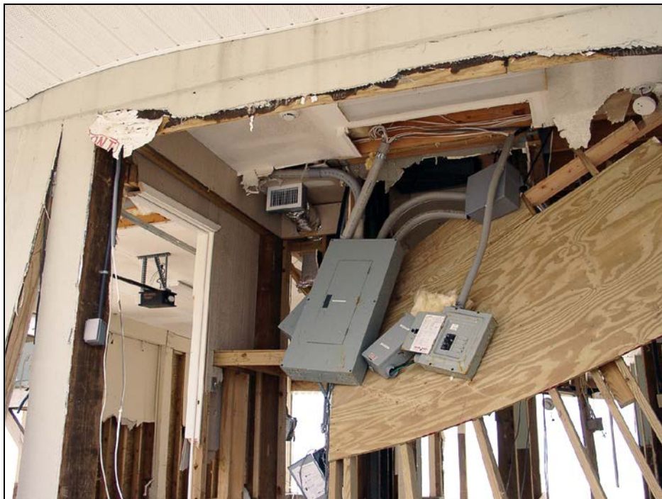
Figure 13: Utilities mounted on wall, which prevented the wall from breaking away cleanly
