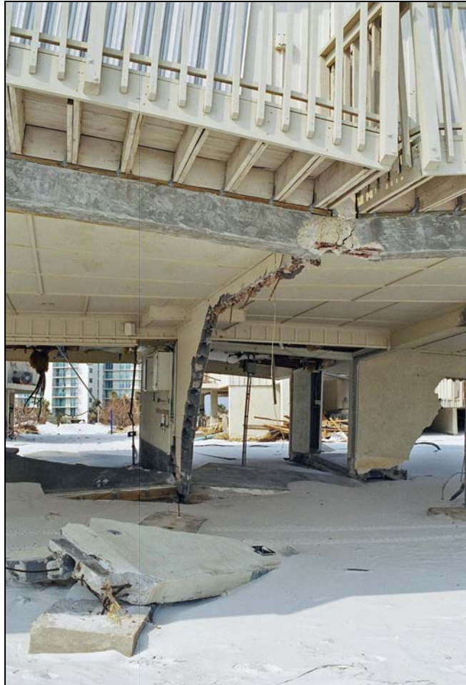
Figure 19: Failure of a shore-perpendicular solid foundation wall that supported a low-rise building, which resulted in failure of the beam and floor system that were supported by the shore-perpendicular wall
