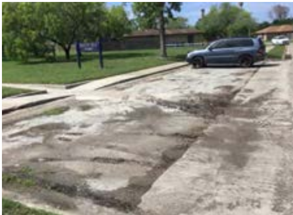
South Seas Park. Many off-street parking areas are in need of substantial surfacing improvements.
