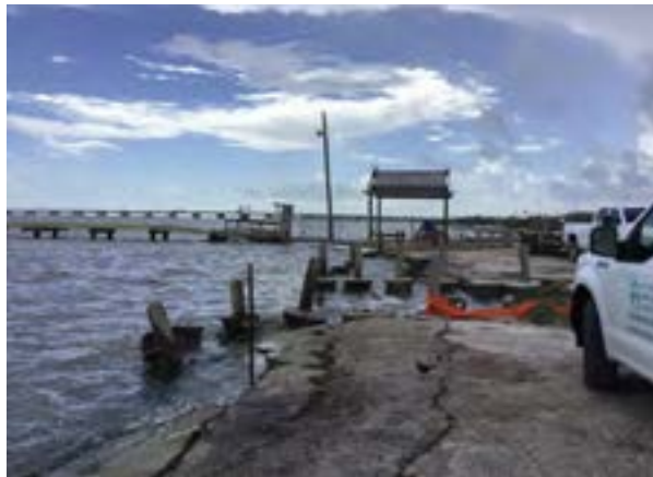
The Dimmit Fishing Pier site is in an advanced stage of deterioration and requires shoreline stabilization.
