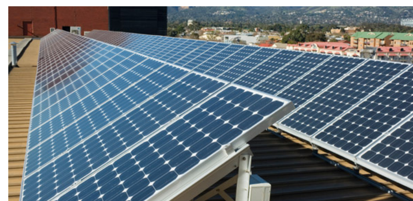
Static Photovoltaic Array
