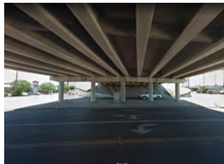
Existing Underpass Conditions, potential site for a gateway art. Source: Google Maps
